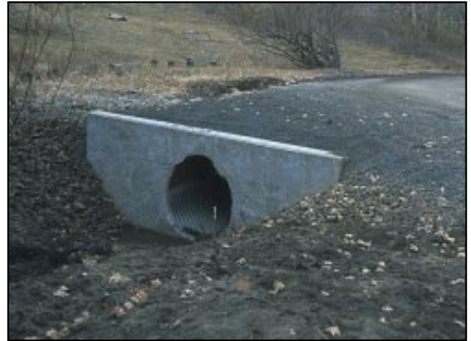
Photo 4.6 A well designed and installed culvert with head walls for efficiency and fill protection.
