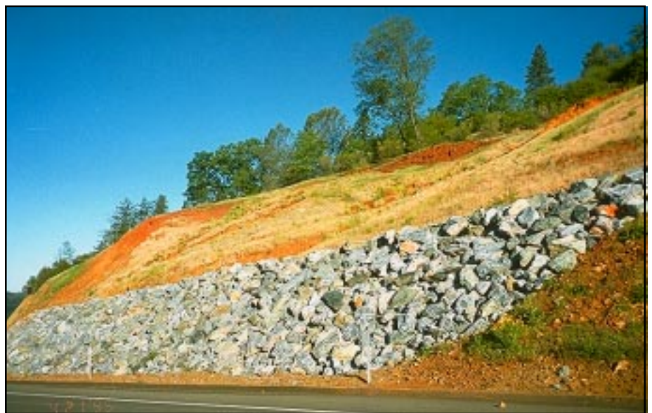
Photo 11.7 A drained rock buttress can be used to stabilize a cut slope failure area.
