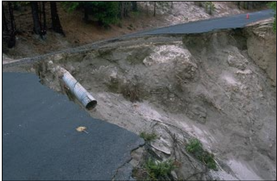
Photo 11.10 A road fill failure in steep terrain which now needs either a retaining structure or a large road cut around the failure.
