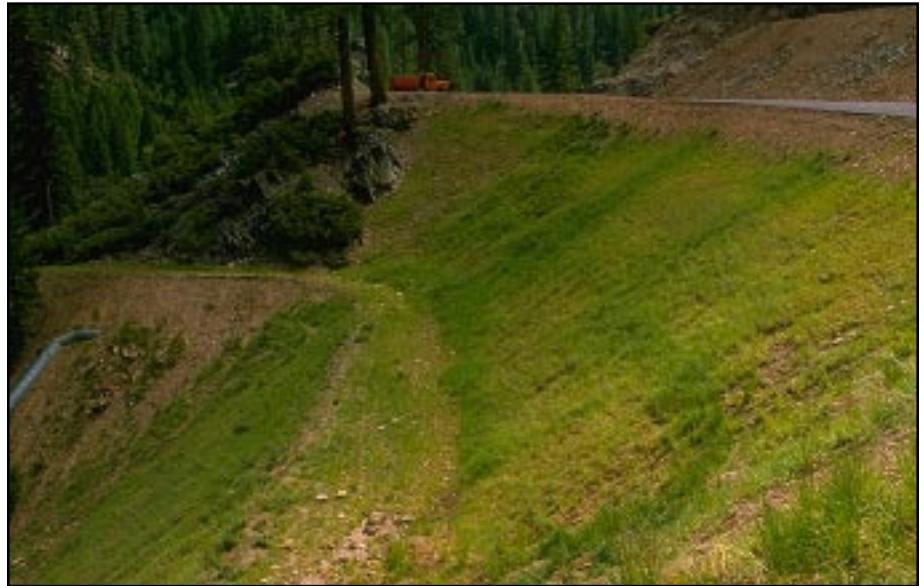
Photo 11.5 Construct fill slopes with a 1 1/2:1 or flatter slope (to promote vegetation growth) and stabilize the fill slope surface. Use benches (terraces) on large fill slopes to intercept any flow of surface water.
