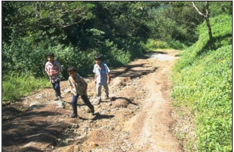
Photo 2.4 Adverse environmental impact from road surface erosion caused by steep road grades and insufficient cross-drains. This road is also difficult to maintain.
