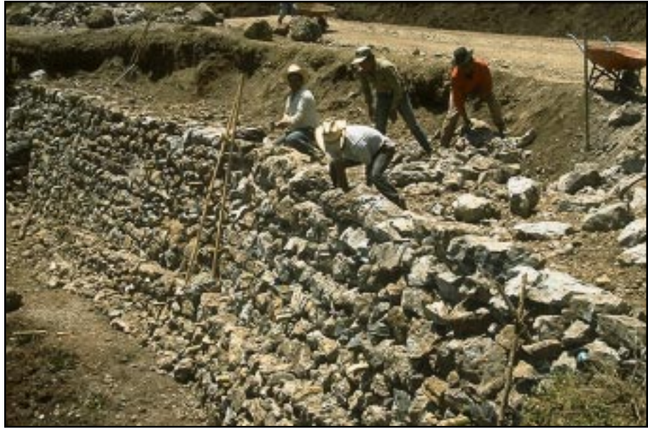
Photo 11.8 Use physical slope stabilization methods, such as retaining walls, reinforced fills, or rock buttresses where necessary in areas of space limitation on steep slopes.
