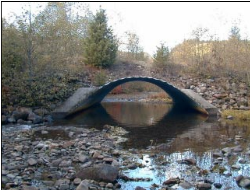
Photo 2.3 A bottomless arch pipe culvert that spans the active stream channel and doesn't constrict the flow, maintains a natural stream bottom, and helps promote fish passage. (Photo provided by S. Wilson-Musser)
