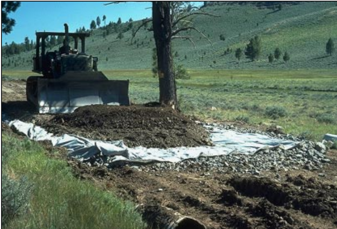
Photo 7.10 Use subdrains or filter blankets when necessary to remove groundwater from the roadway subgrade in local wet or spring areas. Note that this design needs a second layer of geotextile between the soft subgrade soil and the coarse filter rock to keep the rock clean.
