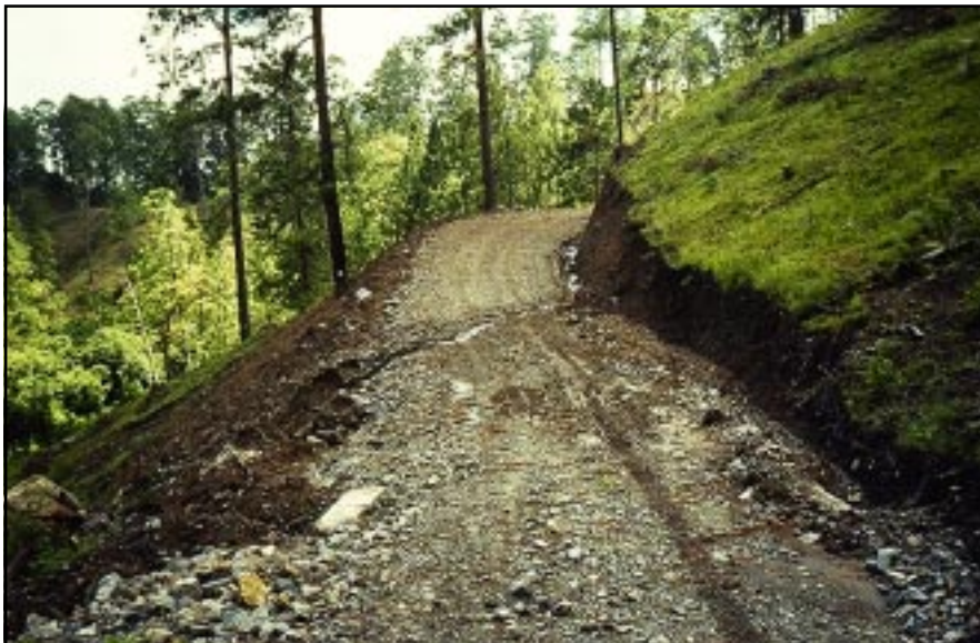
Photo 4.3 Avoid constructing roads with steep grades or on steep side slopes. It is difficult to control drainage with steep road grades.
