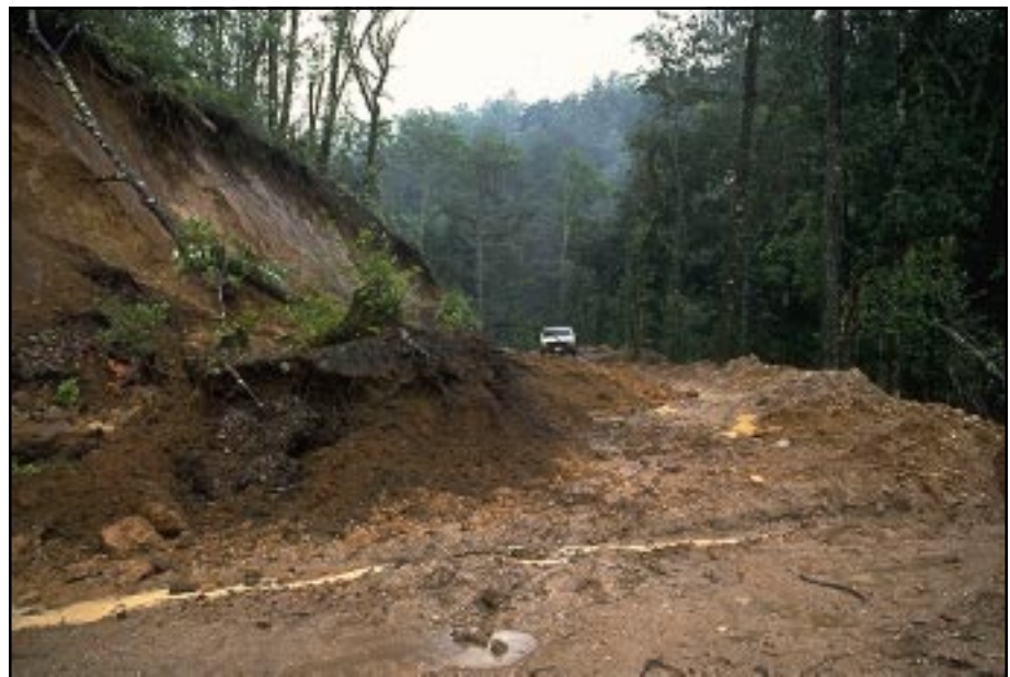
Photo 1.3 A problematic road because of roadcut failures. Instability problems cause road user delays, and high maintenance or repair costs.
