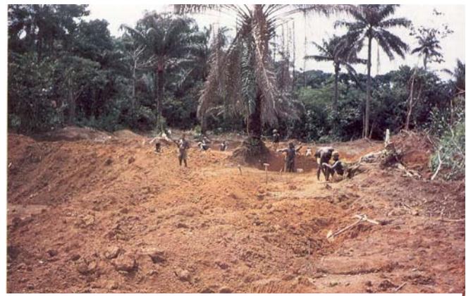
As-dug, nodular laterite. Can this be used as base for a LVR? Definitely, YES, when used in the right context (e.g. min. embankment height, sealed shoulders, compaction to refusal, etc. see photo. below)
