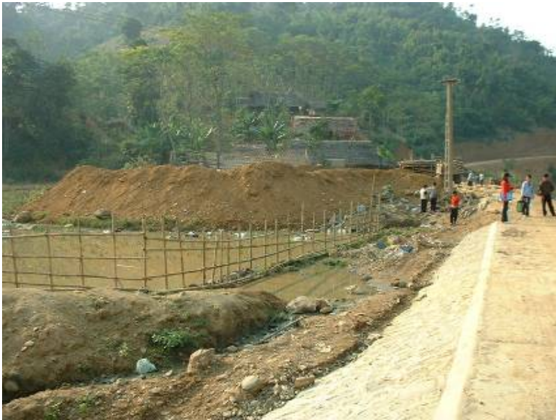
Picture 4.1: Local people show the research team an unstable section of a WB financed road where a culvert should have been built (Phu Tho)
