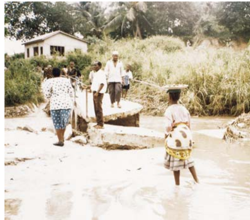
Photo 8.5-2. Damaged bridge after heavy rains
