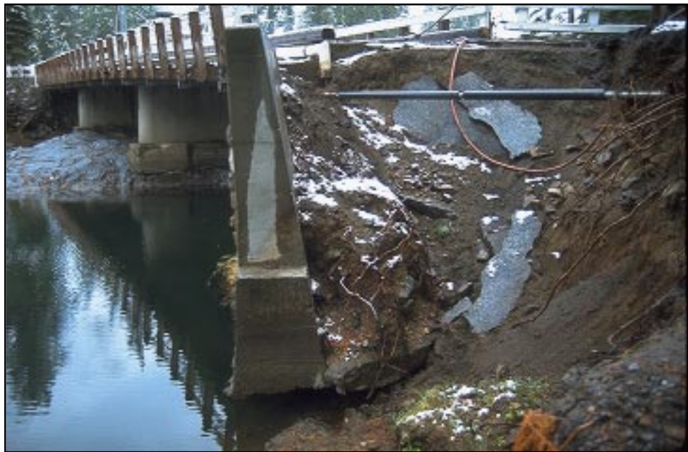
Photo 6.1 Scour behind a bridge abutment caused by insufficient channel and stream bank protection during a flood.
