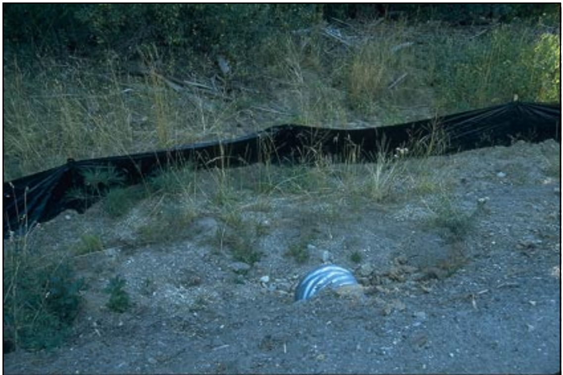
Photo 6.6 Use of a geotextile as a “silt fence” to trap sediment from a construction area.
