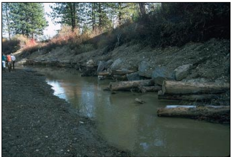
Photo 6.3 A root wad, log, and rock armored stream bank built for protection against scour. Logs and vegetation can offer an attractive alternative to riprap in relatively low stream velocity areas.
