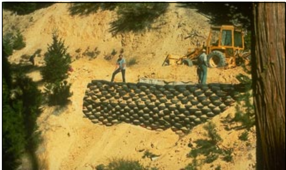
Photo 11.11 A tire-faced, mechanically stabilized earth (MSE) retaining wall, with layers of geotextile reinforcement, being used to gain road width in a fill failure area. MSE (reinforced soil) structures are often the least expensive retaining structure available. Welded wire MSE walls are also commonly used.
