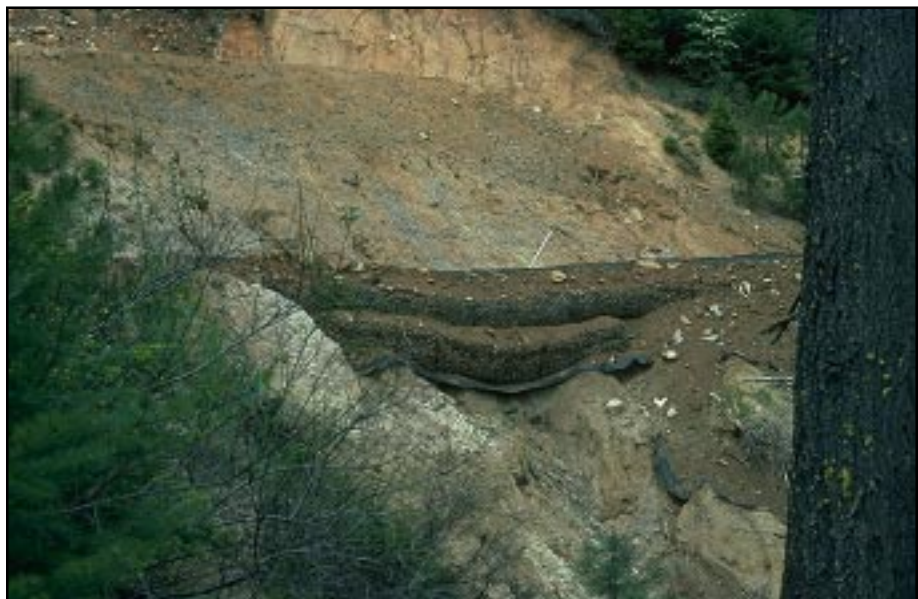
Photo 11.12 A gabion retaining structure which will fail soon due to lack of a suitable foundation. All retaining structures, either mechanically stabilized earth (MSE) walls or gravity walls, require a good foundation .
